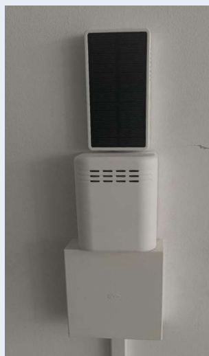
EnoSense® CO2 sensor with Energy Harvesting solar panel (top) and EnoSense® Radon (bottom), installed in a teaching area at the University of La Laguna.
