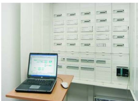
Fig. 6: LON service room
