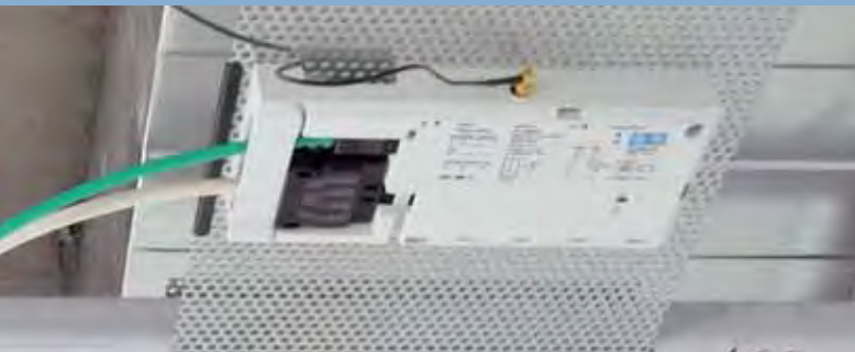
Wieland gesis RC EIB/KNX gateway with external antenna beneath a ceiling.
